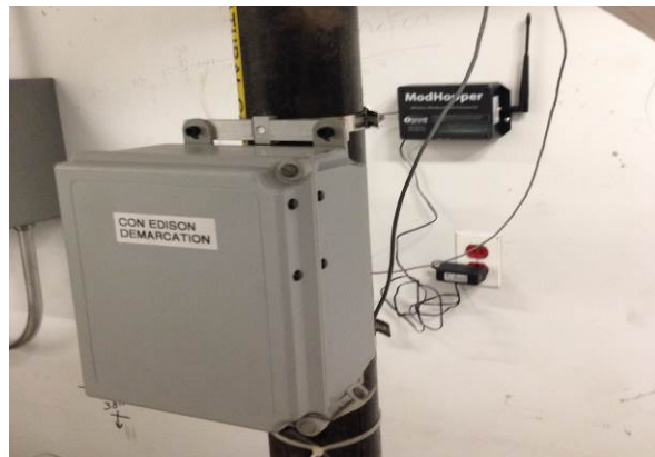
Con Ed demarcation enclosure (right) and Mod Hopper wireless transmitter (right) – located in gas meter room in basement.
