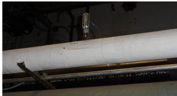
TLS – Recovered heat loop supply temperature.
