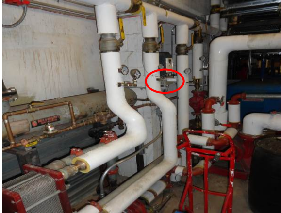
TLR1 – Recovered heat loop temperature after chiller, Con. Ed. steam HX, and space heating HX.
