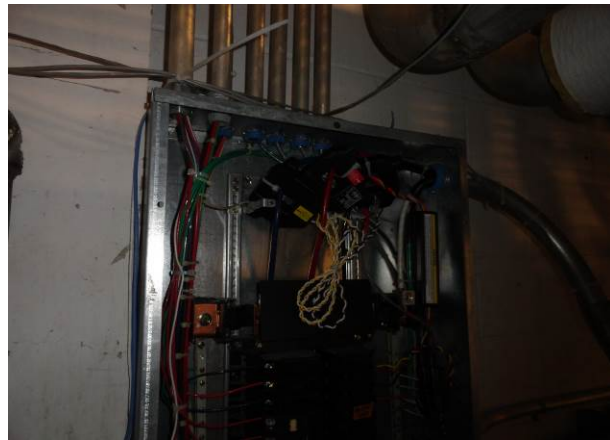
Veris H8035 power meter installed in breaker panel to measure parasitic loads.
