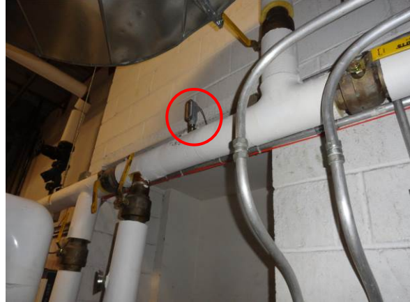
TLR2 – Recovered heat loop temperature after DHW.
