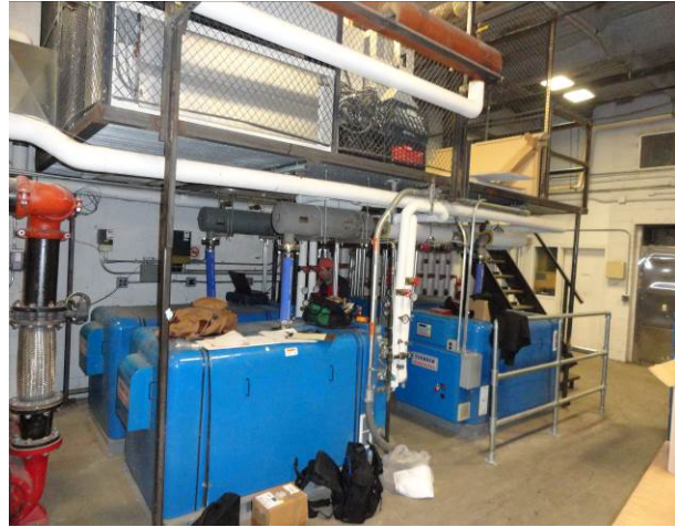
Site view – four (4) CM-60 cogen units, located in loading dock area.
