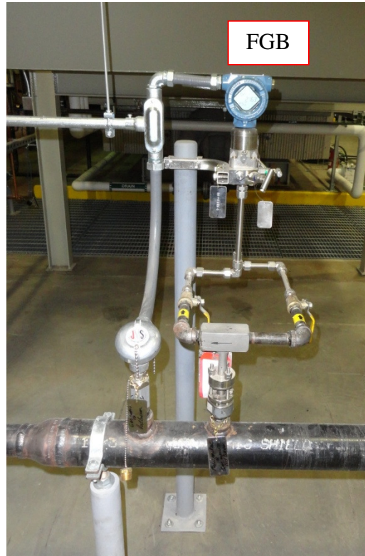
Duct Burner Gas Meter (FGB)
