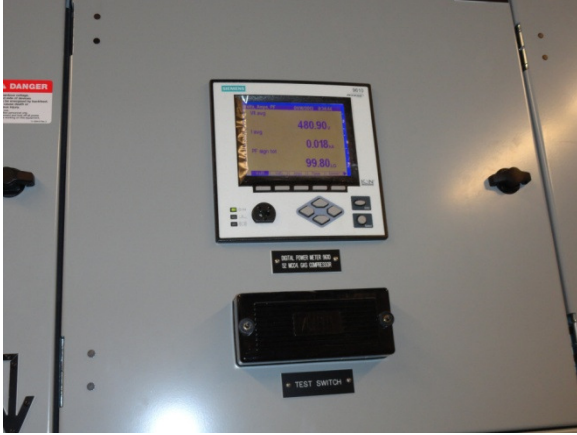
Gas Compressor Power Transducer MCC-4 (WPAR2)
