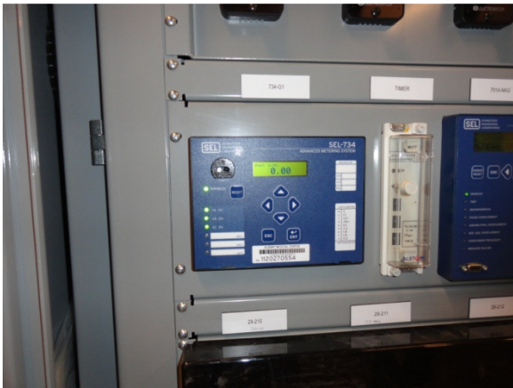
Gas Turbine Gross Output Power Transducer SEL-724 (WG)
