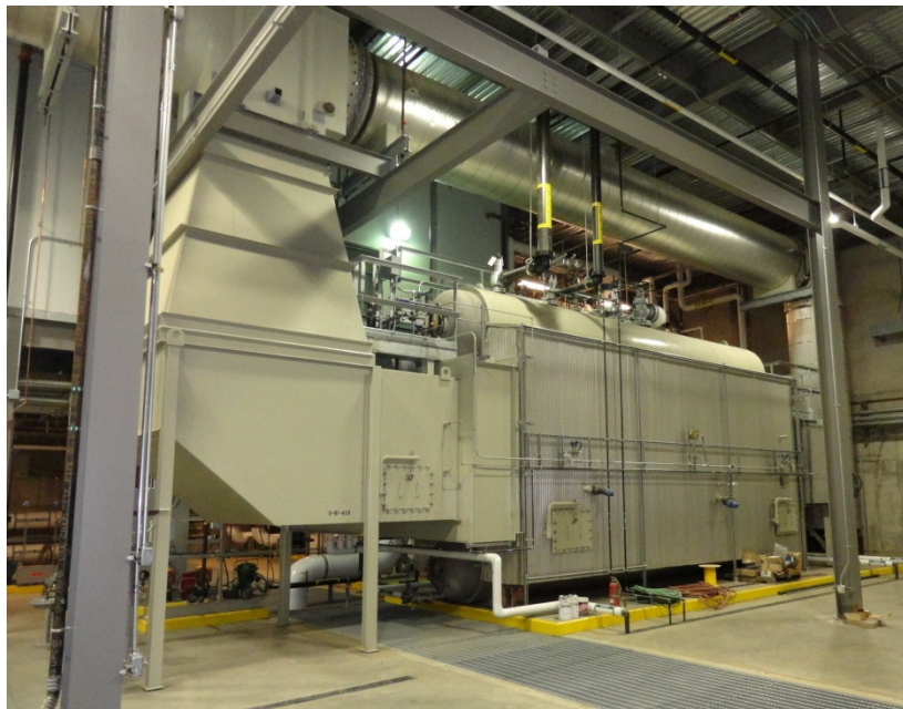
Heat Recovery Steam Generator (HRSG)
