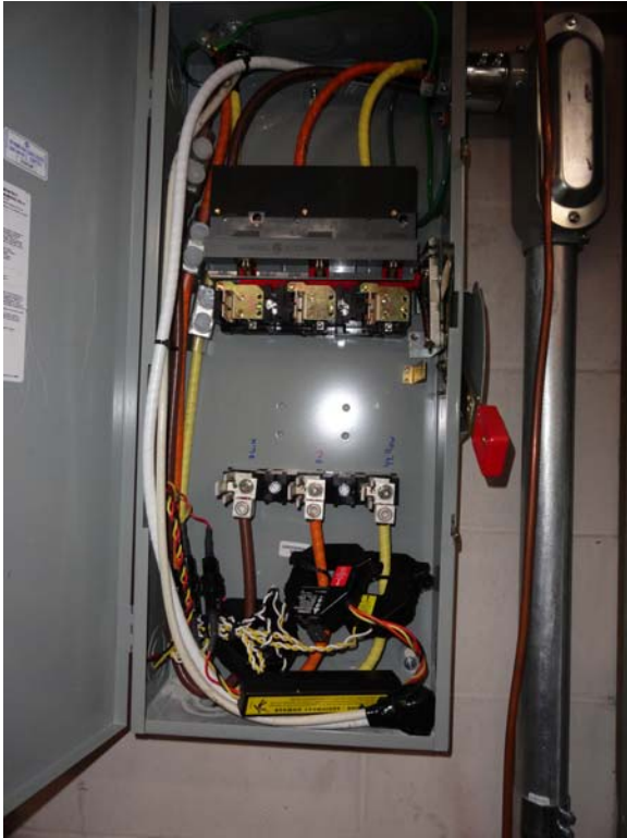
Figure 3. Microturbine Power Transducer Installed in 480 VAC disconnect
