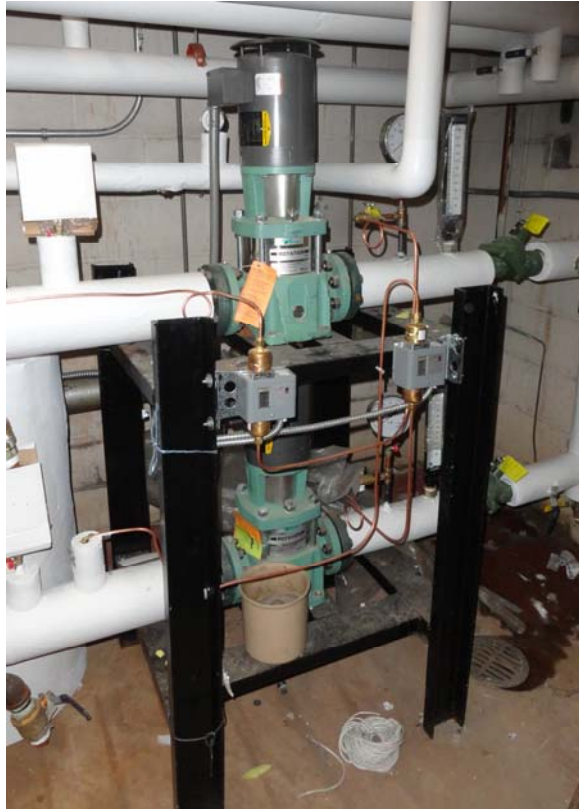
Heat Recovery Loop Pumps
