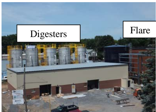
Digester System and Biogas Flare
