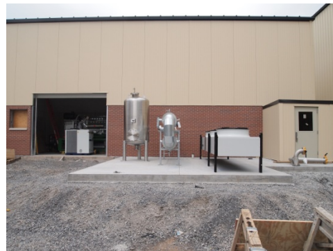
Biogas Conditioning Components
