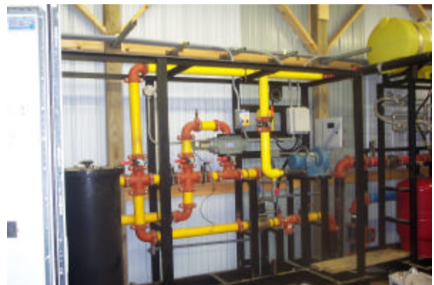
Biogas Conditioning Skid at Emerling
