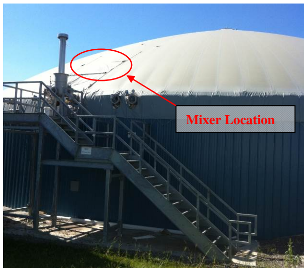
Installed, covered and filled digester, safety vent (left) and mixer location (1 of 4).
