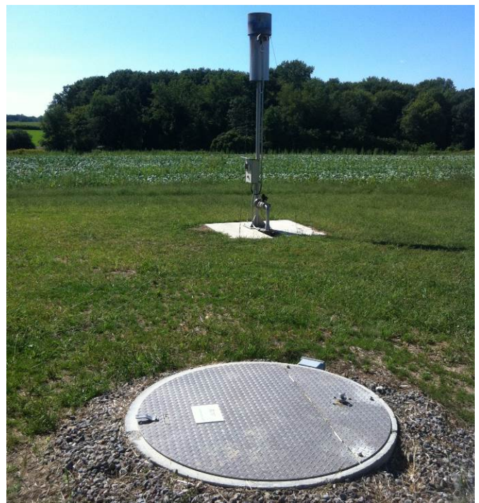
Digester flare (back) and dewatering well (front).
