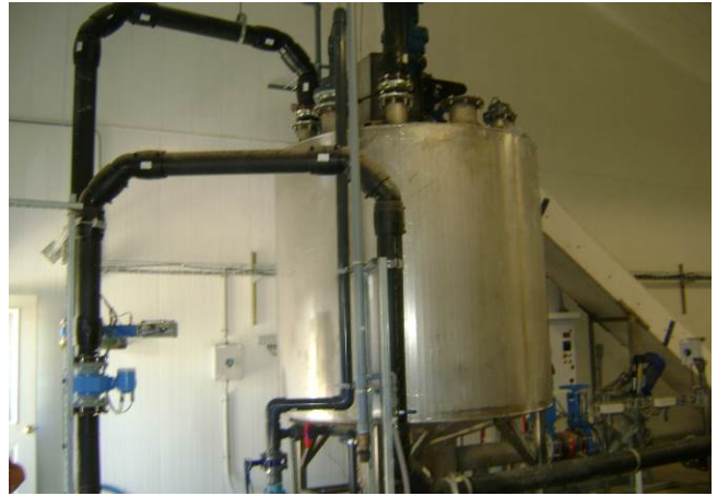
Manure and food or milk waste mix tank – before entering digester.
