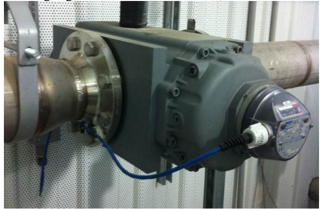
Roots biogas meter – measures total biogas (generator and flare)
