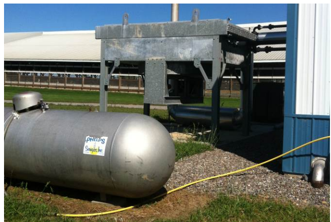
Propane storage tank – only used for boiler at startup.
