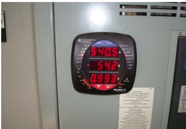
Shark 200 revenue grade power meter, installed in switchgear to right of DIA.NE XT3 engine controller.
