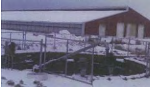
Raw manure collection pit currently installed on farm.
