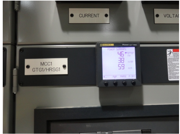
CHP Parasitic Loads MCC-1 (WPAR2)
