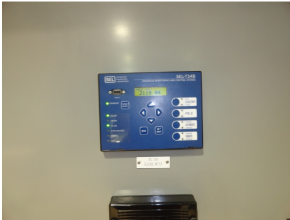
Gas Turbine Gross Output Power Transducer SEL-734B (WG)
