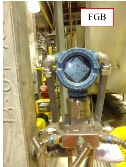
Duct Burner Gas Meter (FGB)
