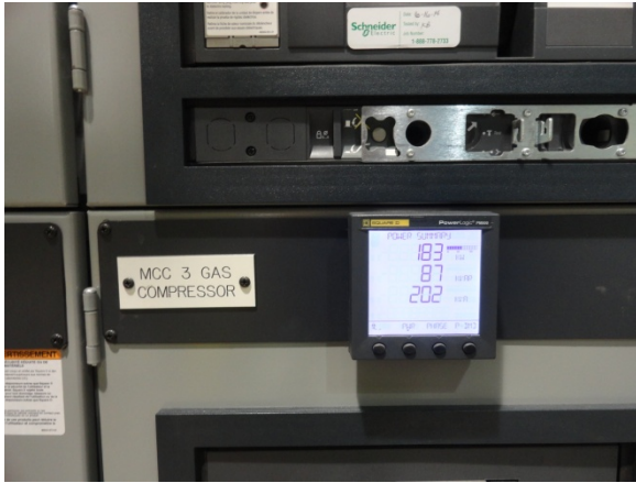
Gas Compressor Power Transducer MCC-3 (WPAR2)
