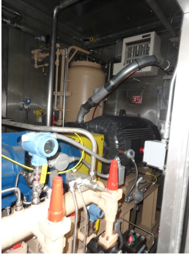
Gas Compressor (in enclosure on roof)
