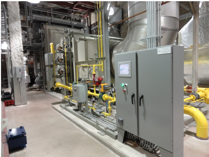
Heat Recovery Steam Generator (HRSG)
