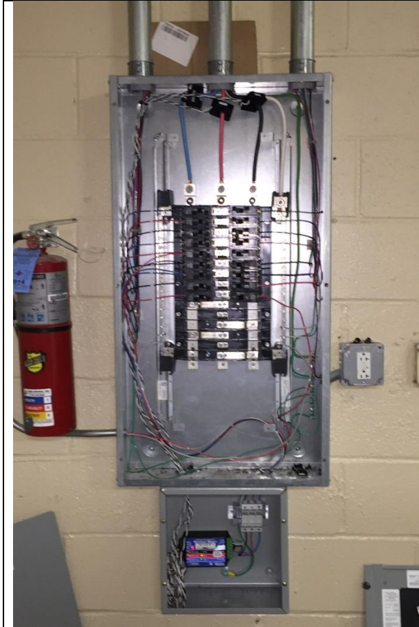
Power transducer below electrical panel with parasitic loads
