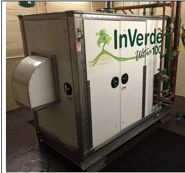
InVerde 100kW cogen unit at 195 Steuben Street
