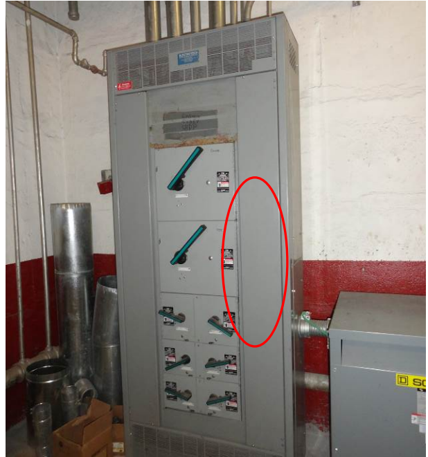
Location of cogen power meter (WG)
