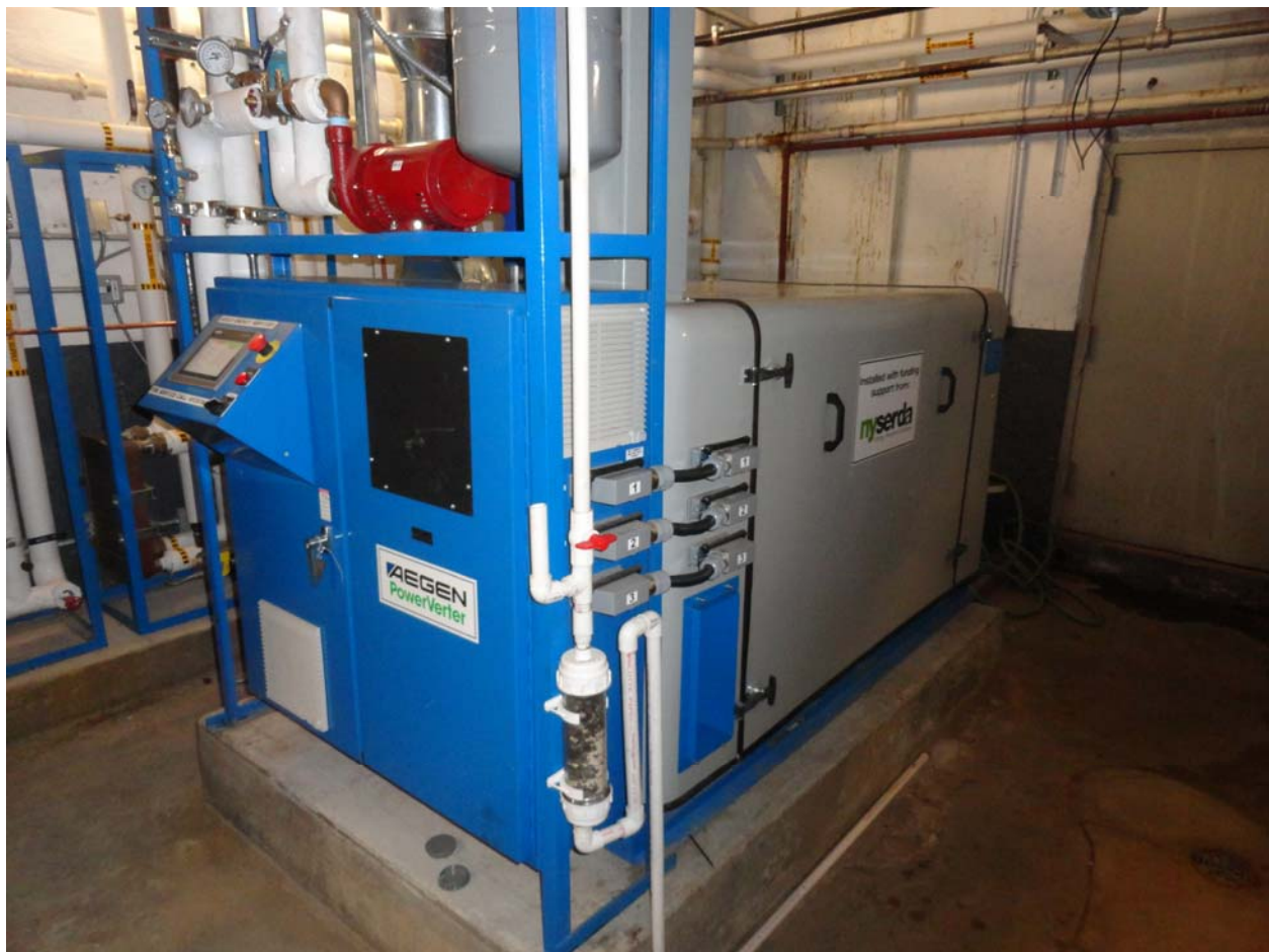
Figure 1. Birchwood Towers – The Kyoto Cogen Unit
