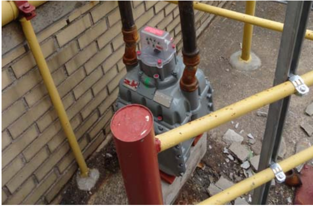
Utility gas meter, located in next to building (FG)
