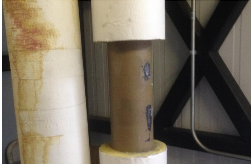
Figure 5. Jacket Water Supply (right) and Return (left) Pipes in the Chiller and HRSG Container
