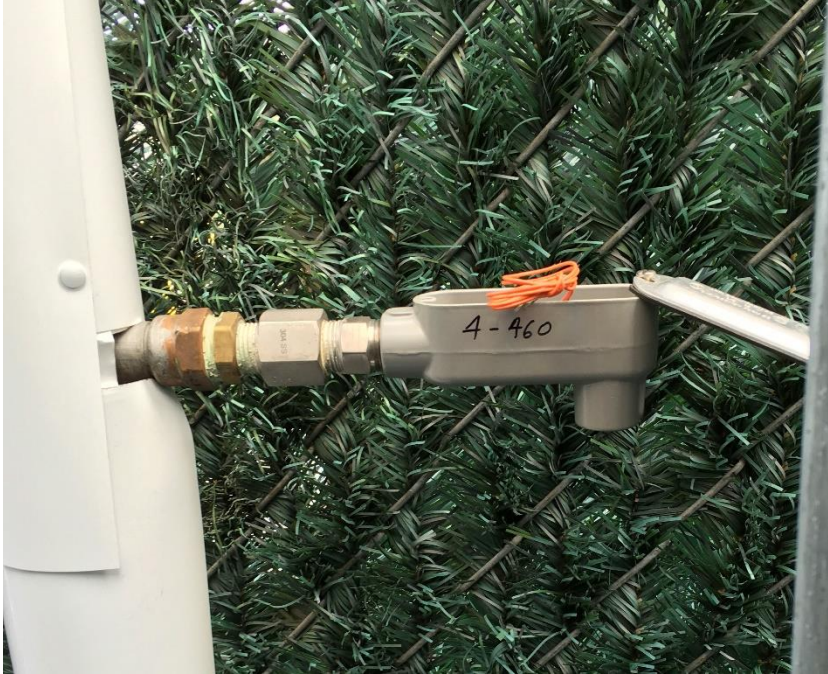
Temperature sensor after the dump radiator (TLR2)
