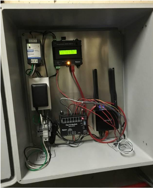
CDH M&V enclosure with Cradlepoint cellular modem in lower right corner
