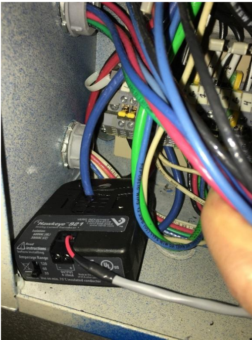
ICCP1 - Located in Cogen Control Panel 1
