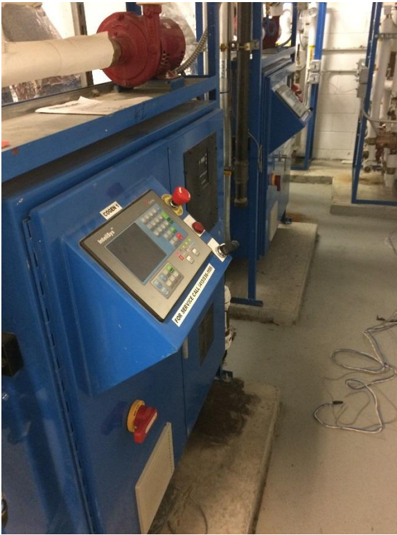
Aegen TP75-LE cogen units located in basement mechanical room.
