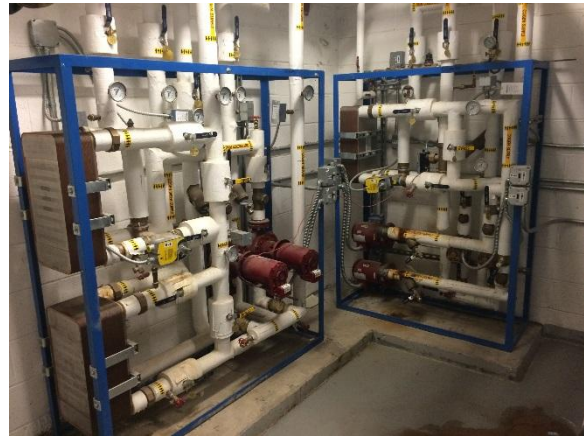
Basement mechanical room HX skid, with Badger 380 BTU meter (CDH to install Veris 10k Type 2 thermistor in well).
