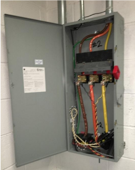
Generator 2 Power Transducer
