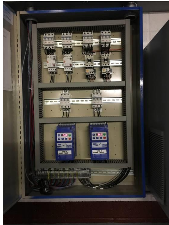
CCP Panel with VFDs and Veris H921 Analog CT
