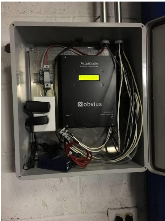
CDH Monitoring Enclosure w/ Obvius Data Logger
