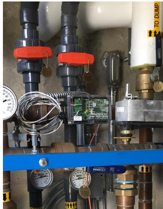
Dumped Heat Load BTU Meter
