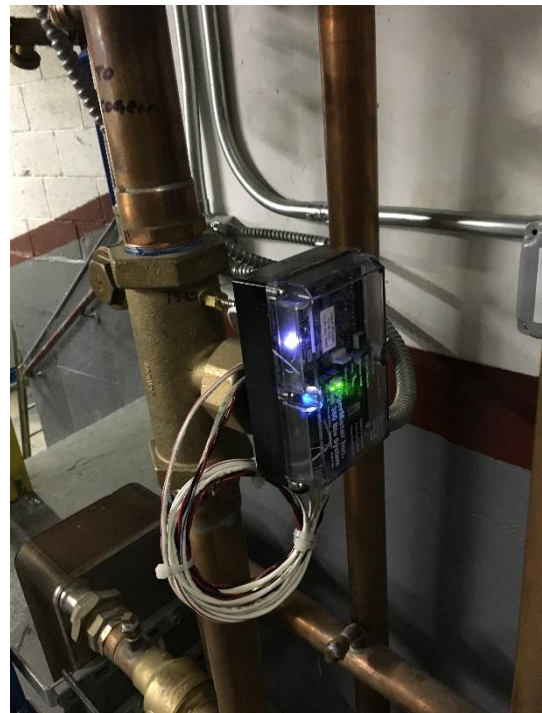
HW Loop BTU Meter (In Boiler Room)
