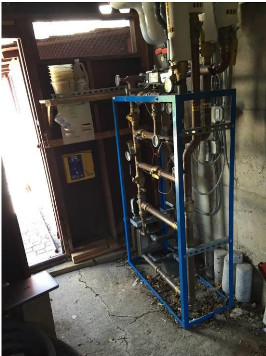
Pool & Dump Skid in Pool Shed with BTU Meter
