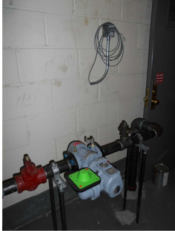
Gas meter, signal wire, no pulse head installed
