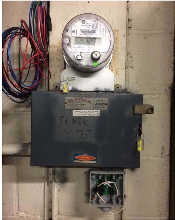
GE utility power meter (top) and demarcation pulse enclosure (bottom)
