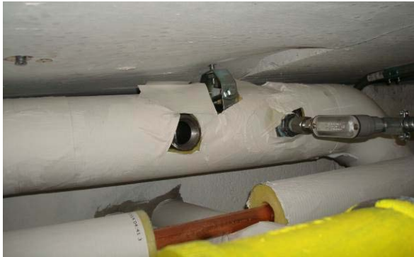
Recovered heat loop supply temperature sensor THW1 (right)
