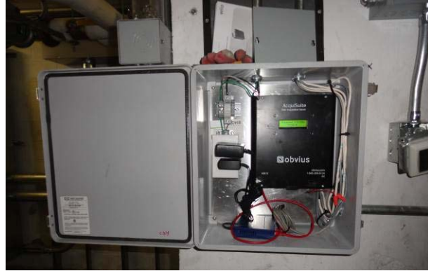
CDH panel containing data logger and CDH network switch.
