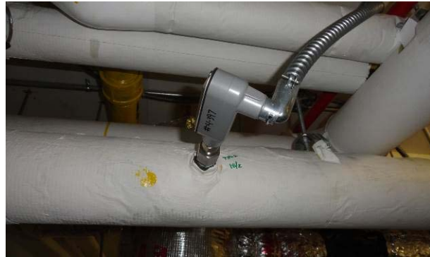
Recovered heat loop temperature THW2 after useful HX
