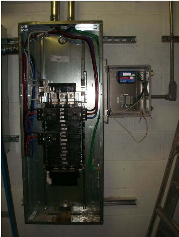
Parasitic load panel (left) and parasitic power meter and enclosure (right)
