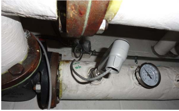
Recovered heat loop return temperature sensor THW3 after dump radiator
