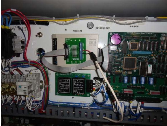
Modbus card (TYP) installed in each InVerde electrical cabinet for gross generator output.
