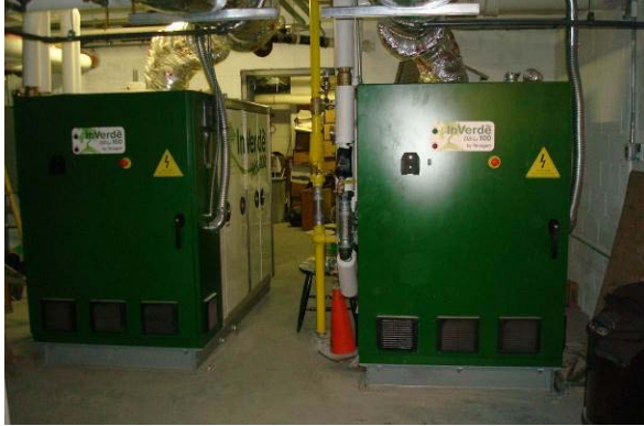
Tecogen InVerde 100 kW cogen units (2x) located in basement mechanical room.
