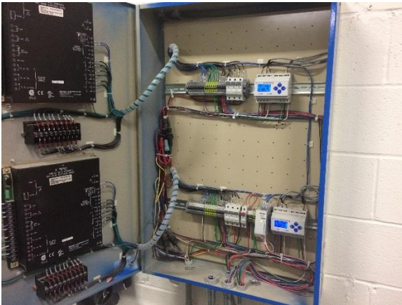
Total facility power meters located in main electric room.
