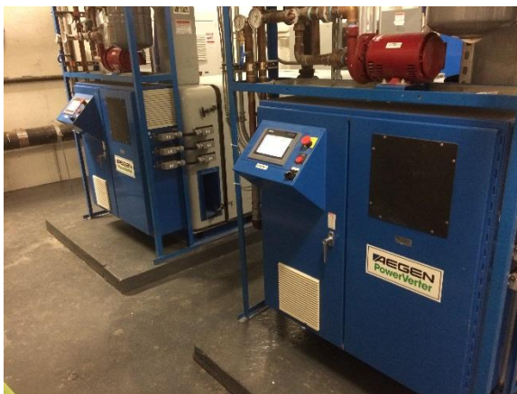
Aegen TP75-LE cogen units located in basement mechanical room.
