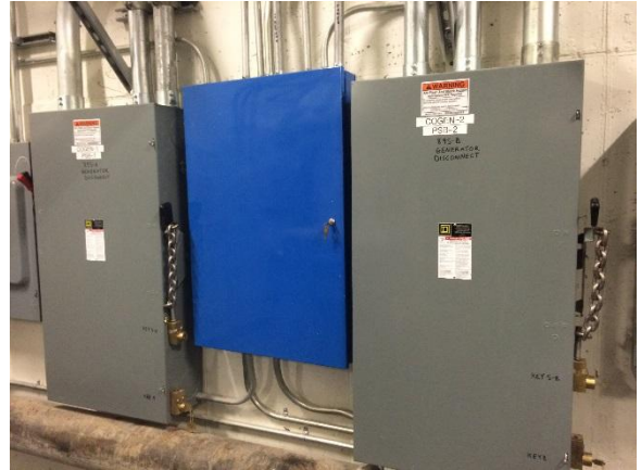
Cogen power meters located in cogen disconnects (grey). Parasitic power meter located in Aegis panel (blue).
