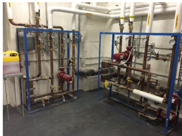
Basement mechanical room HX skids, with Badger 380 BTU meter (left) and Veris 10k Type 2 Thermistor (right).
