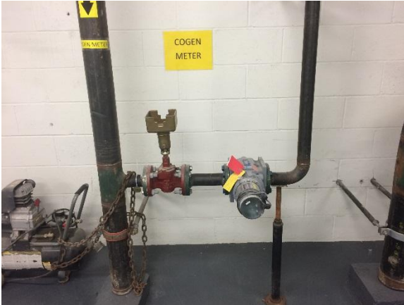
Utility gas meter located in gas meter room.
