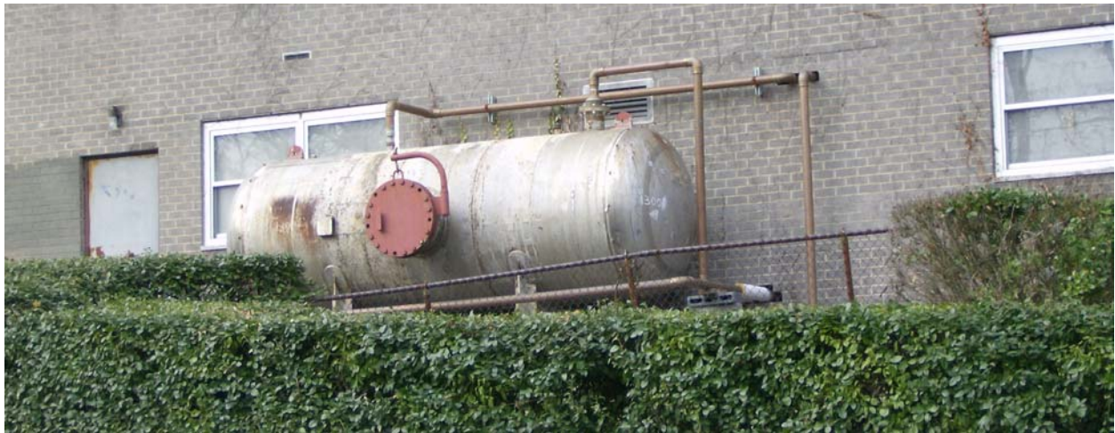
3,000 gallon DHW Storage tank added at the back of the building
