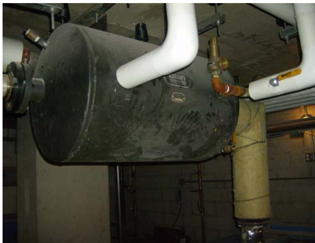
Cain Exhaust Heat Recovery HX
