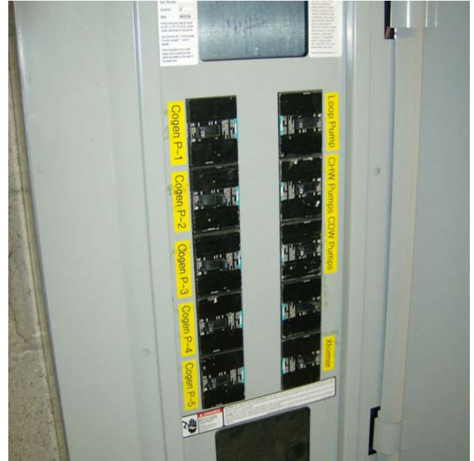
480 V Electrical Panel (parasitic loads)
