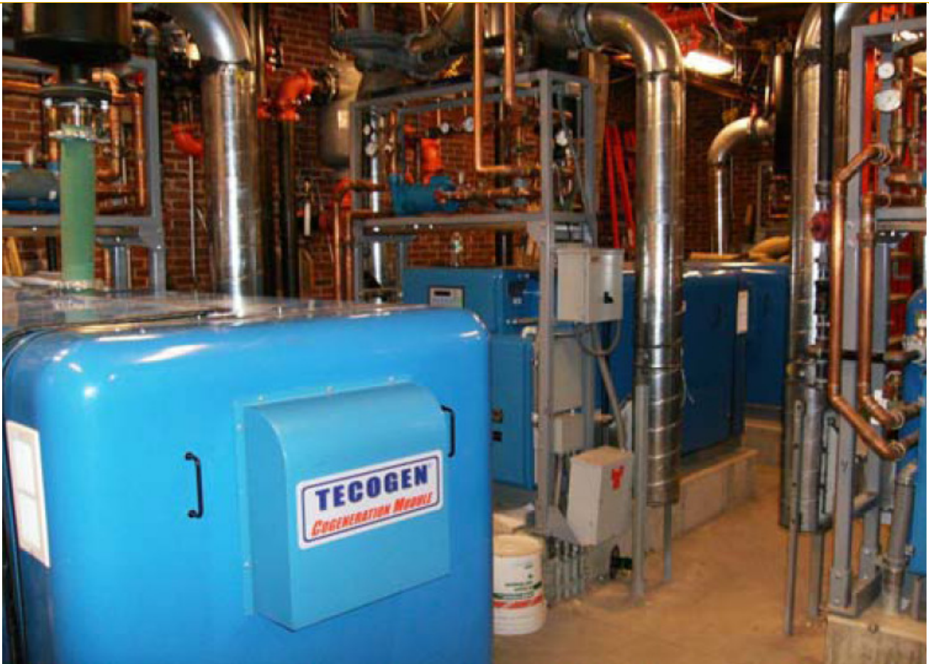
FIGURE 4 MECHANICAL ROOM SHOWING SEVERAL ENGINE GENERATORS
