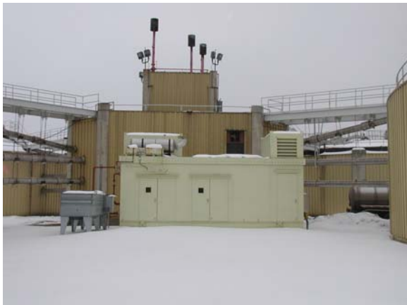
Foreground: CHP Enclosure & Radiator Inter-cooler. Background: Digester Control House & Waste Burners (Flares)
