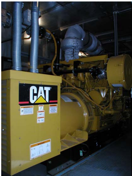
Caterpillar 380 kW Engine/Generator Skid
