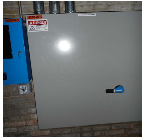
Cogen contactor panel - location of gross generator power meter (WT)
