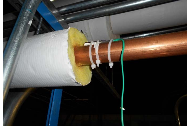
Veris 10k Type 2 Surface Thermistor (THW3), located in boiler room above cogen unit.
