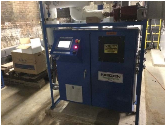
Aegen TP75-LE cogen unit located adjacent to sub-basement boiler room.
