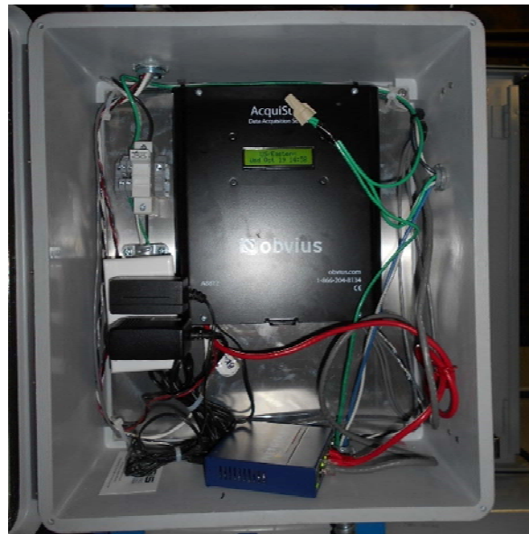
CDH panel containing data logger and CDH network switch.
