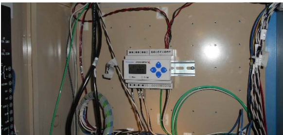
Veris E50 total facility power meter (WB) located next to cogen contactor panel.
