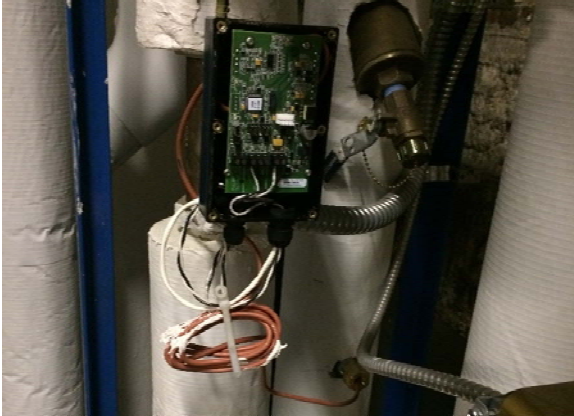
Badger 380 BTU meter (THW1, THW2, FHW).
