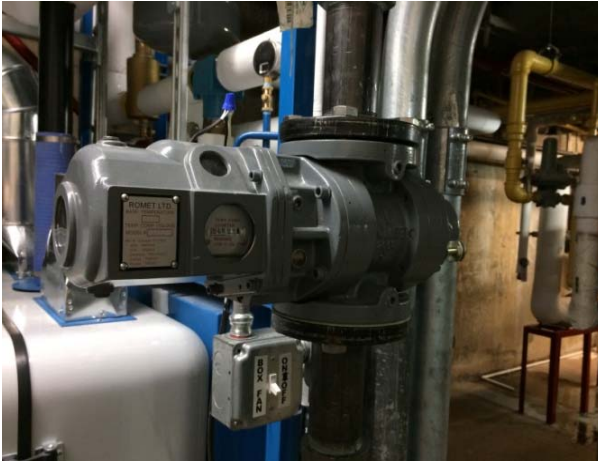
Romet RM2000 gas meter (FG) located in the boiler room.
