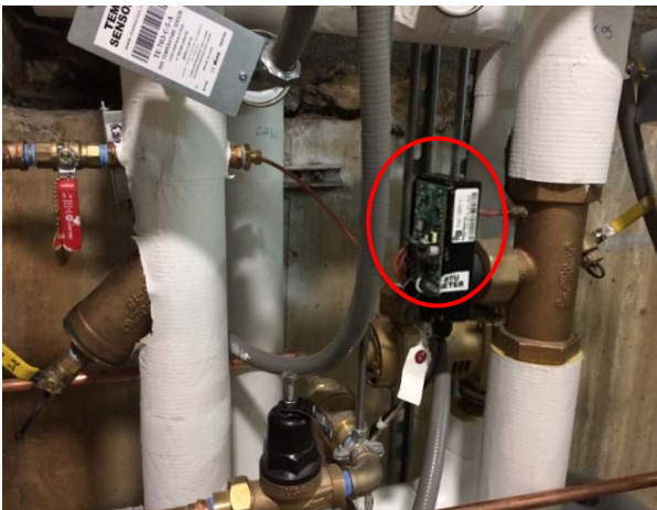
Badger 380 BTU meter on DHW module across useful HX1 (THW1, THW2, FHW) in the boiler room.
