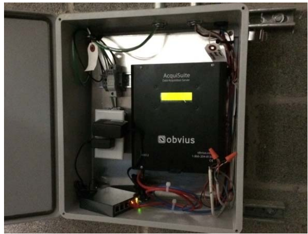
CDH panel containing data logger and CDH network switch located in the boiler room.
