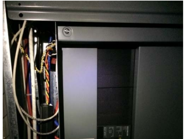
Parasitic power meter (WP) located in SBDP-A subpanel on level two of the parking garage above the boiler room.
