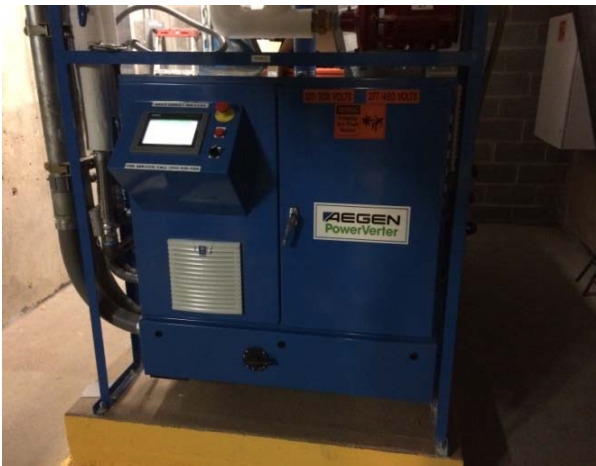
Aegen PowerVerter 100 kW cogen unit located in the boiler room.
