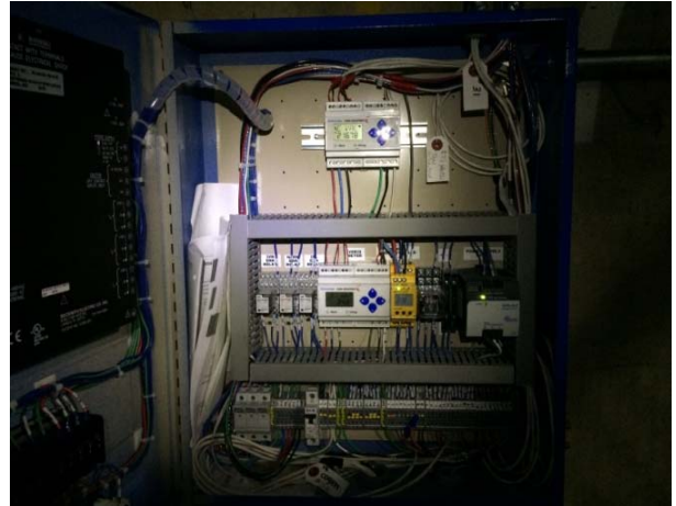
Veris E51 total facility power meter (WB1 & WB2) in Beckwith panel on level two of the parking garage above the boiler room.
