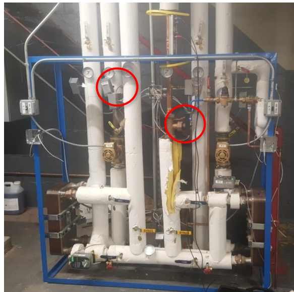
DHW Skid - Located in boiler room Left - Supply BTU temp. sensor (THW1). Right - BTU meter and temp. sensor after useful HX1 and HX2 (FHW ,THW2).
