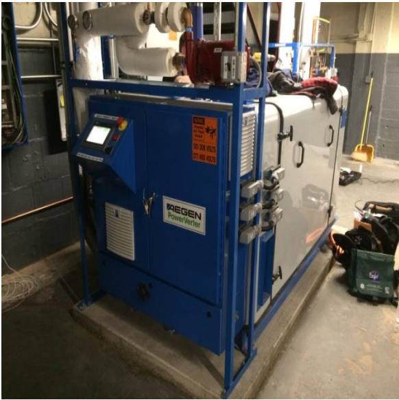
Aegen PowerVerter 75 kW cogen unit located in the boiler room.
