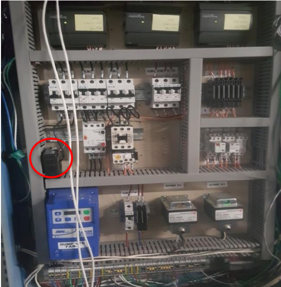
Veris H921 dump radiator current sensor (IVFD) located in Aegis cogen control panel.
