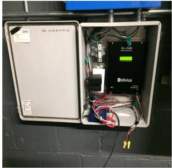
CDH panel containing data logger and CDH network switch located next to unit in the boiler room.
