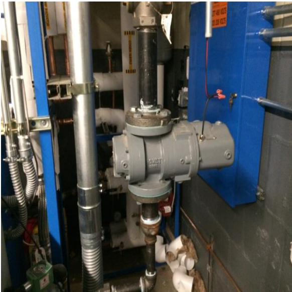
Romet RM2000 gas meter (FG) located in the boiler room next to cogen unit.
