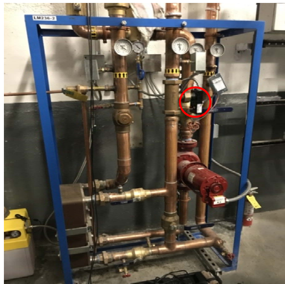
Badger 380 BTU meter on Dump Radiator skid across HX2 (THW2, THW3, FHW) located in the boiler room.
