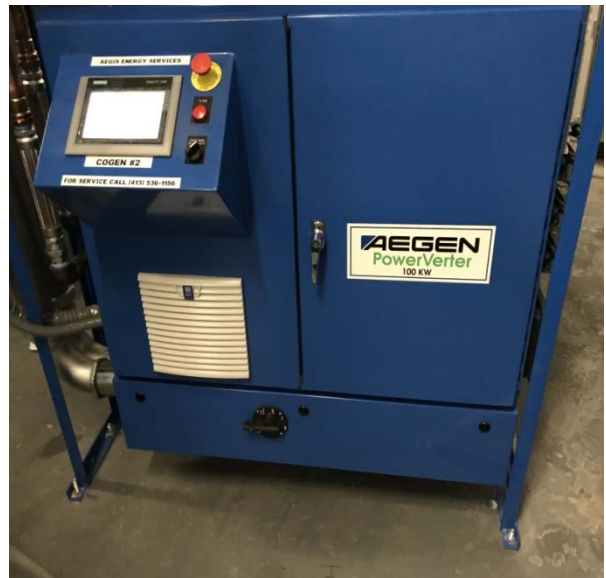
Aegen PowerVerter 100 kW cogen unit #2 located in the boiler room.
