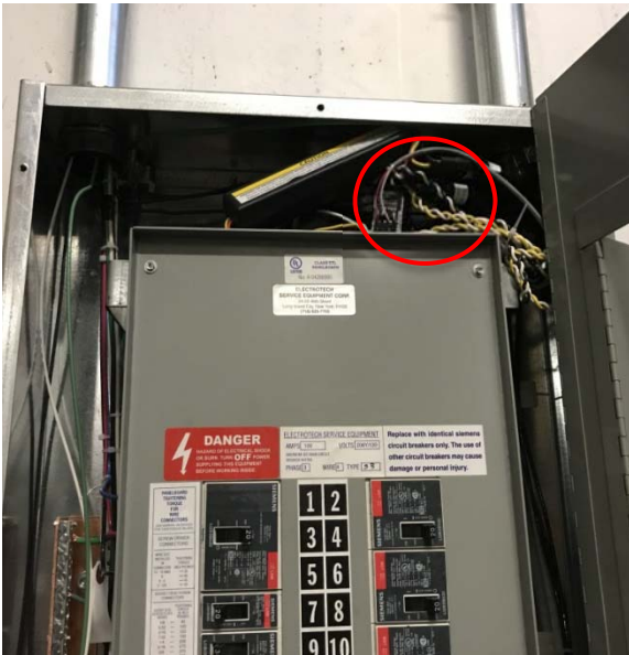
Parasitic Power Meter (WP) installed SBDCG distribution panel. Located above the CDH panel in the boiler room.
