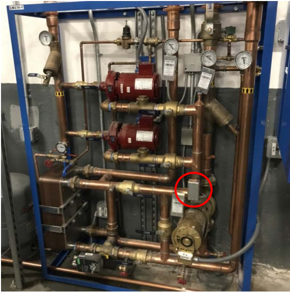
Veris 10K Type II Thermistor (THW1) on DHW skid before HX1 located in boiler room.
