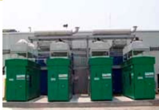
FIGURE 3 INSTALLED GENERATOR MODULES
