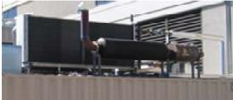
FIGURE 4 DETAIL OF A TYPICAL RADIATOR AND SILENCER
