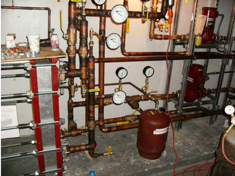
Figure 2. Plate Frame HX, Glycol and DHW Piping
