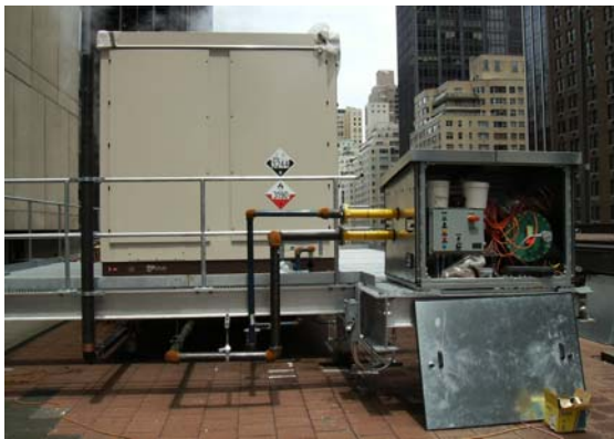
UTC Power Fuel Cell and Gas Booster
