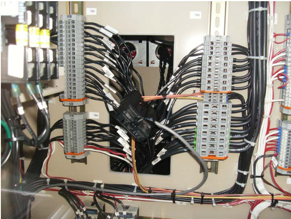
Figure 10. Dry Cooler Current Sensor Located in Fuel Cell Electrical Section
