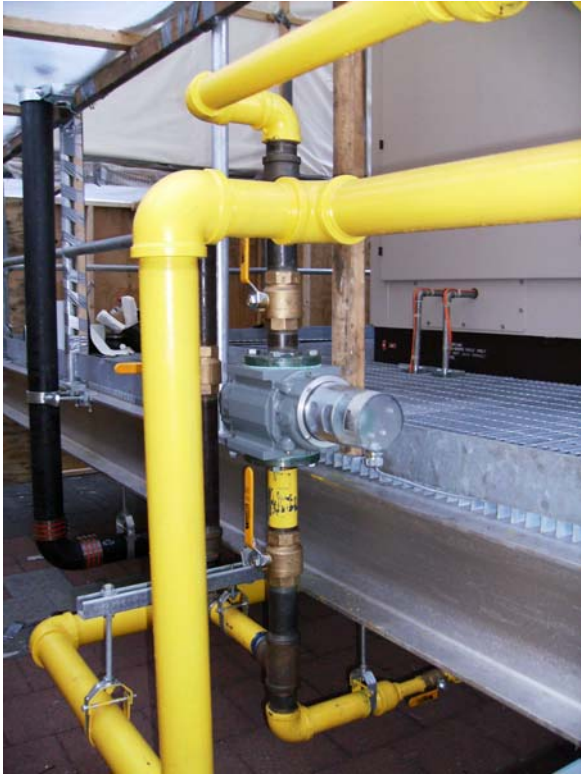
Figure 8. Fuel Cell Natural Gas Meter on 2-inch High Pressure Line
