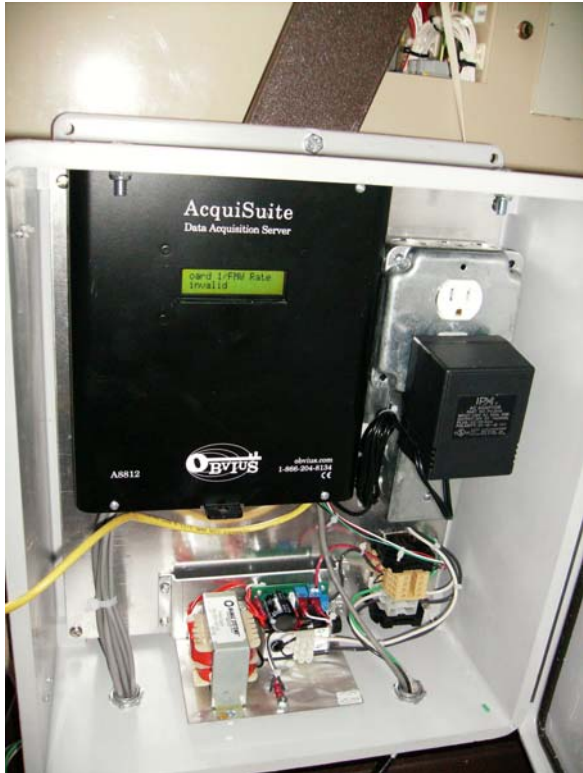
Figure 12. Interior of Data Logging Panel
