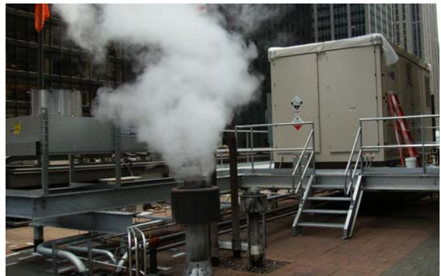
UTC Power Fuel Cell and Dry Cooler
