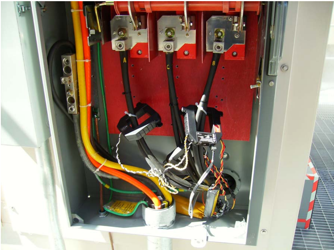
Figure 7. Power Transducer Located at Fuel Cell Unit 400-amp Disconnect
