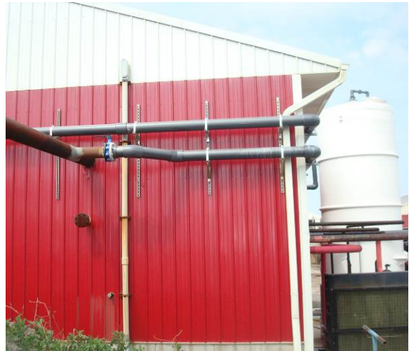
Biogas from digester to scrubber (bottom pipe), and biogas return from scrubber / supply to engine (top pipe).
