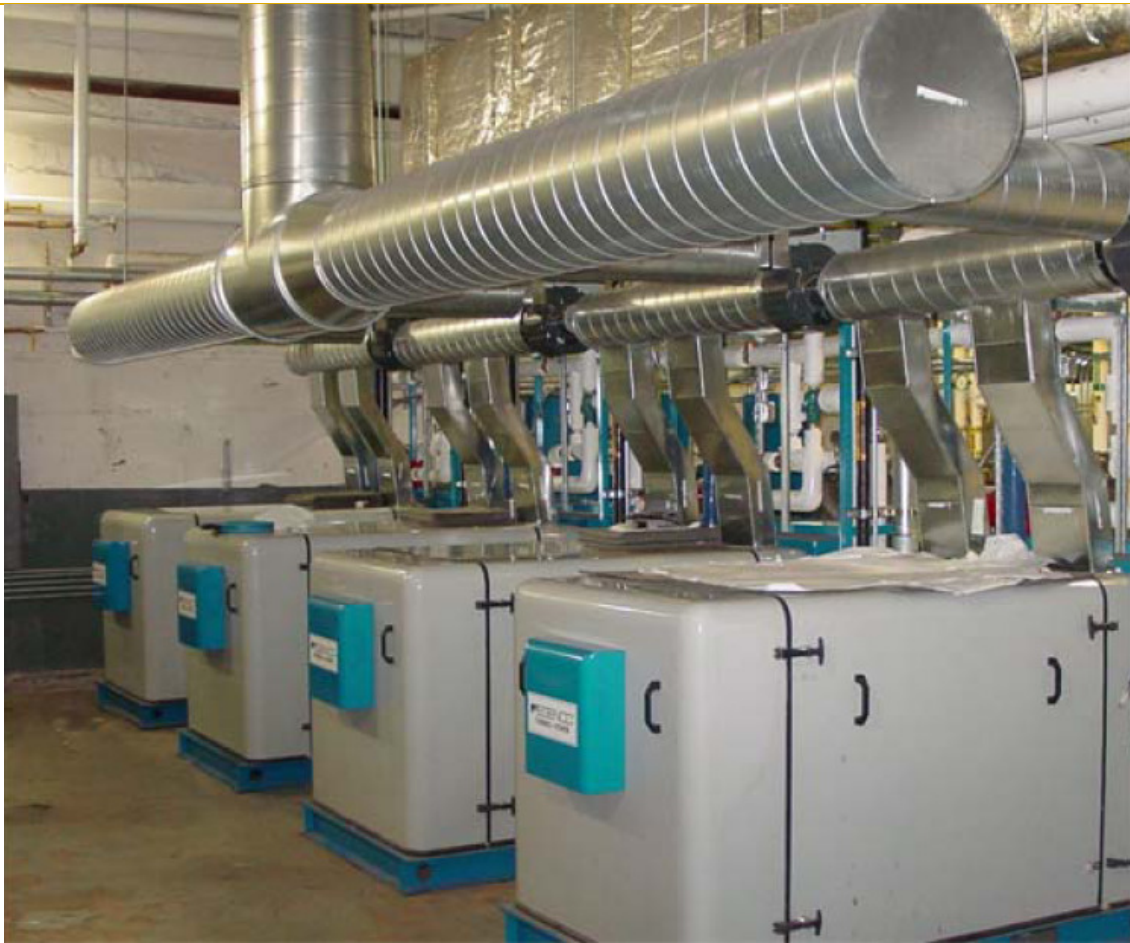
FIGURE 4 FOUR 75 KW ENGINE GENERATORS
