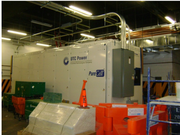
Front of fuel cell, from basement parking lot
