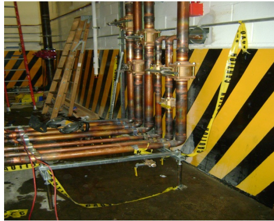
Piping from back of fuel cell: high temp water, low temp water, and cooling water loops
