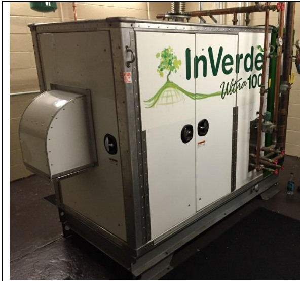
InVerde 100kW cogen unit at 195 Steuben Street
