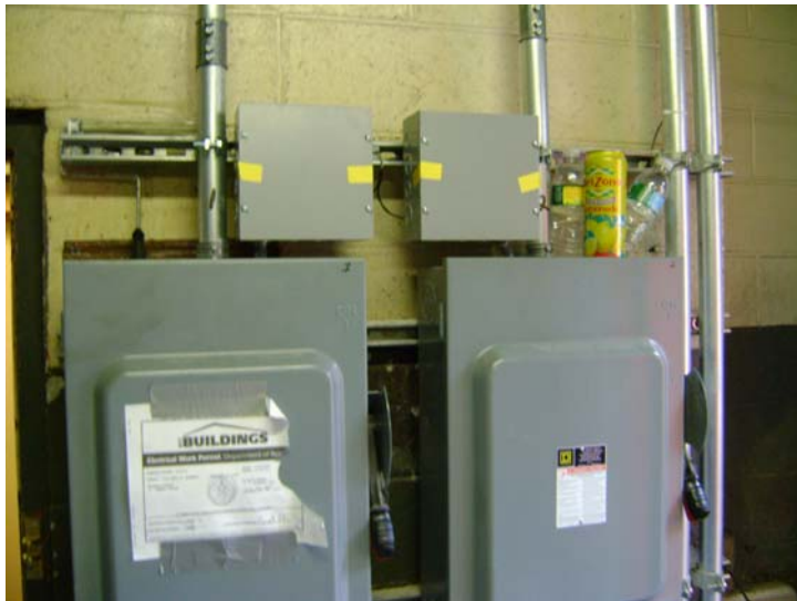
Power Transducer Enclosures near Generator Disconnects (WG1 & WG2)
