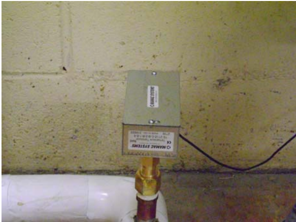
THS – On HX wall, lower left most temp sensor, on bottom pipe.
