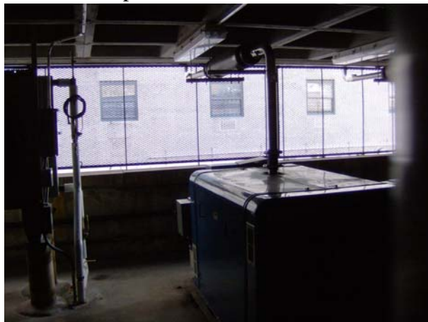
Turbine and generator, on 2 nd floor of parking garage.
