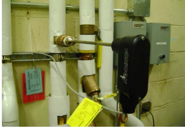
FW – In HX room on left hand wall, above blue pump.
