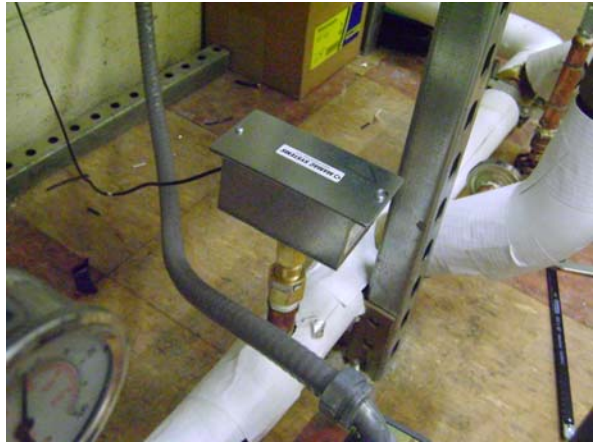
THM – On HX wall, on bottom pipe, center of the three temperature sensors.
