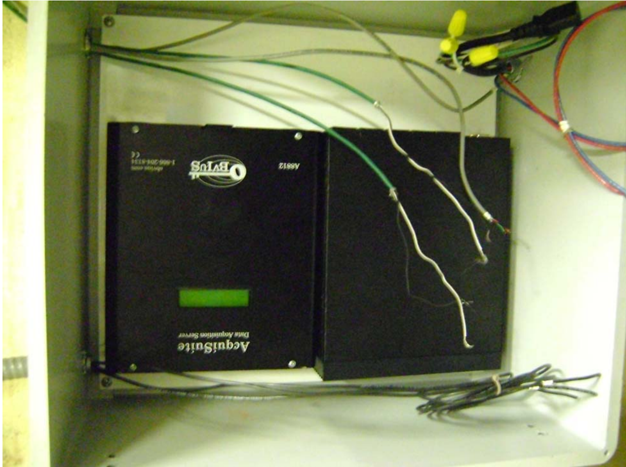
Figure 6. Datalogger and Power Supply
