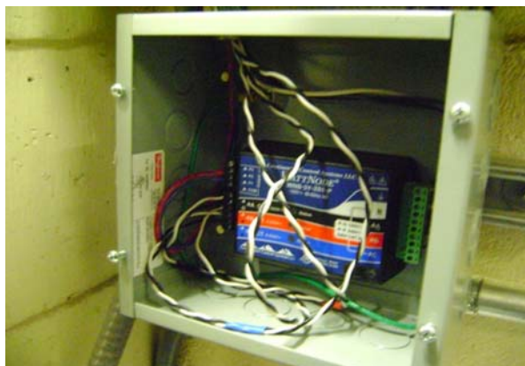
WP – In HX room on left hand wall.
