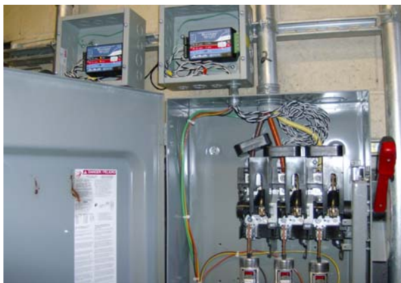
WE1 & WE2 – In front maintenance room where facilities phone lines split.
