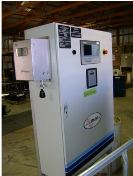
GenCon II Panel w/ Power Meter – NEW ENGINE (WG2)
