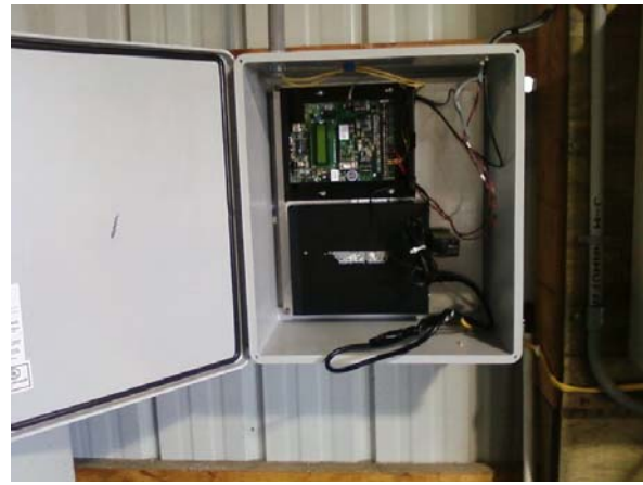
Obvius AcquiSuite data-logger and box.
