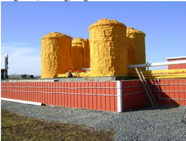
H 2 S Scrubbers
