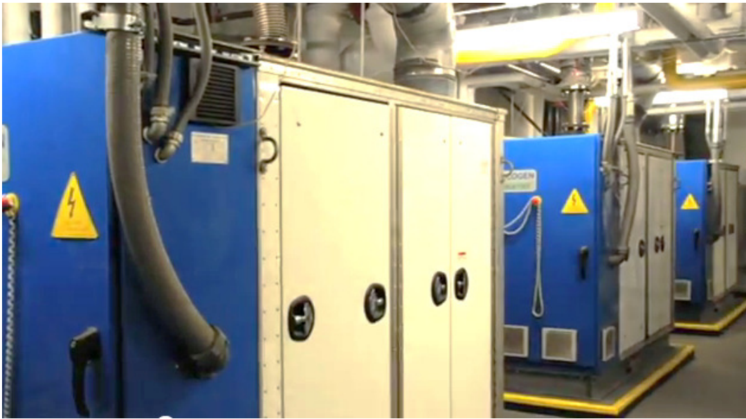
FIGURE 3 THREE OF THE FIVE TECOGEN CM – 100 COGENERATION UNITS
