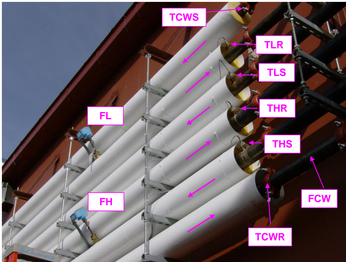
Figure 5. Locations of Temperature and Flow Sensors on Rear Wall of the Facility
