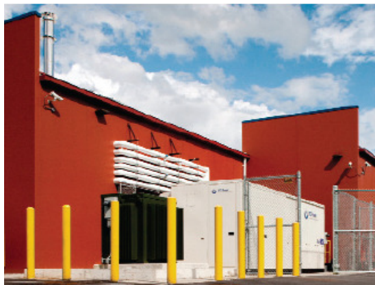
FIGURE 3 FUEL CELL INSTALLED REAR OF THE STORE
