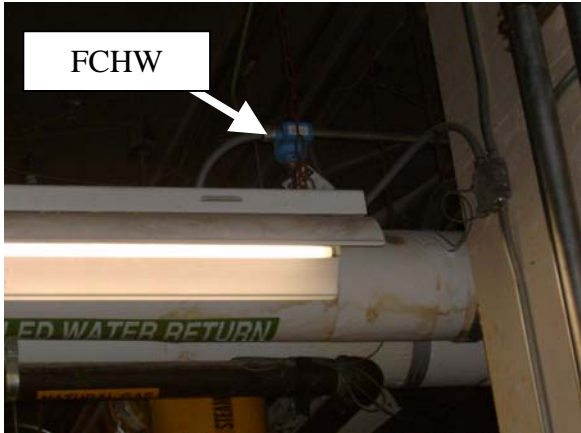
Chilled Water Piping and Location of FCHW sensor
