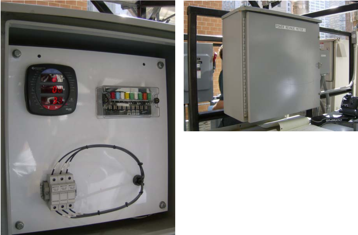
Figure 7. Shark 100 Power Transducer Located Each Turbine Array (typ)
