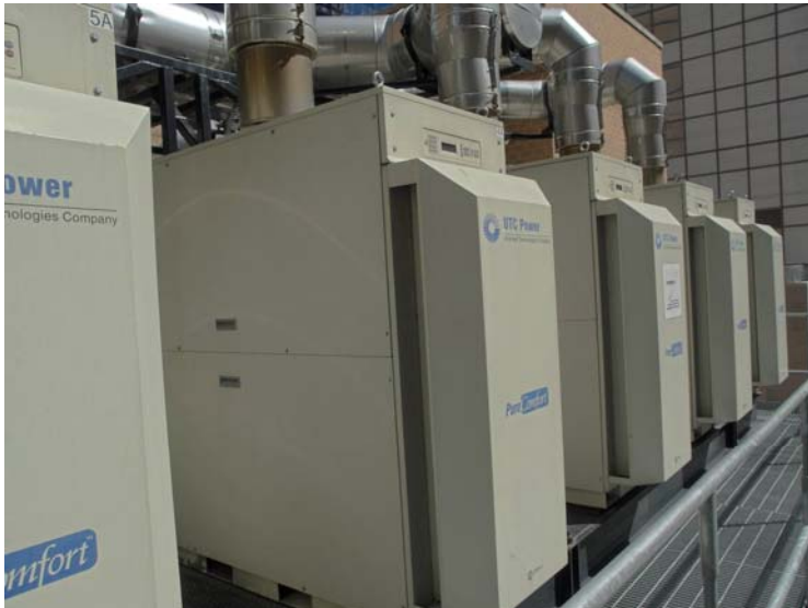
PureComfort Microturbines (System A) – 5 Units
