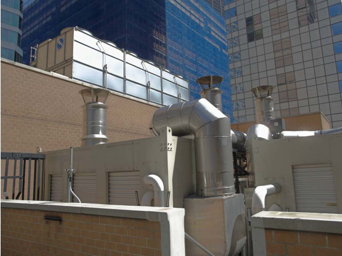
Figure 2. PureComfort System Chillers and Cooling Tower
