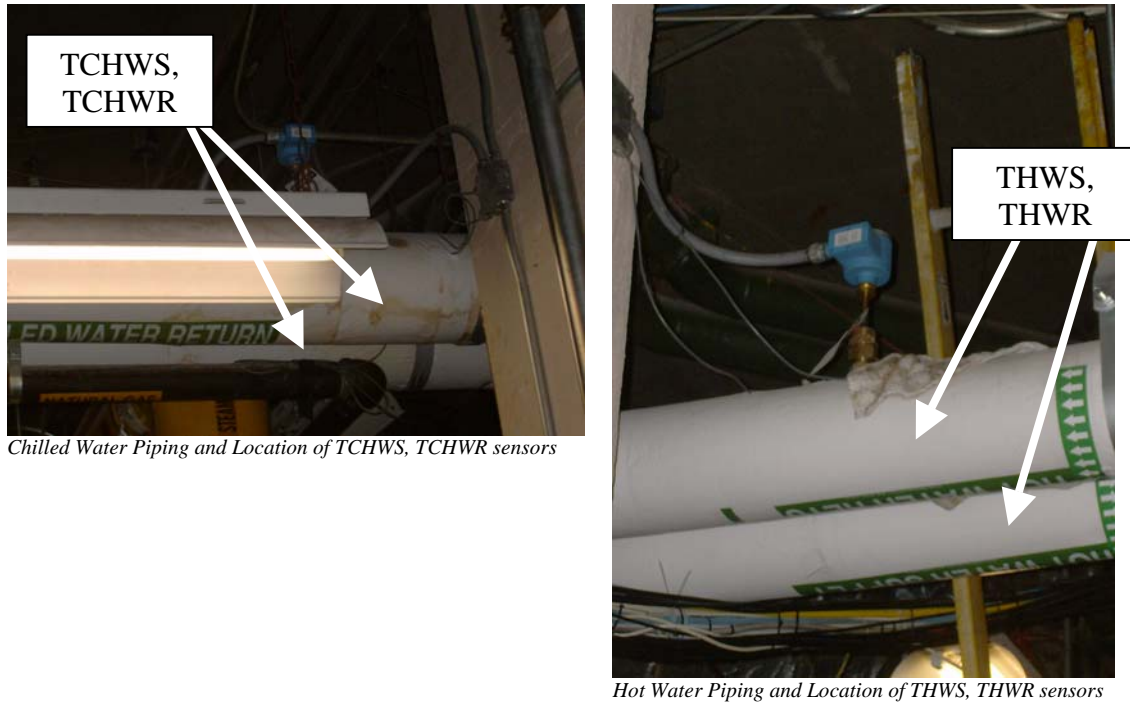
Figure 5. Loop Temperature Sensor Locations
