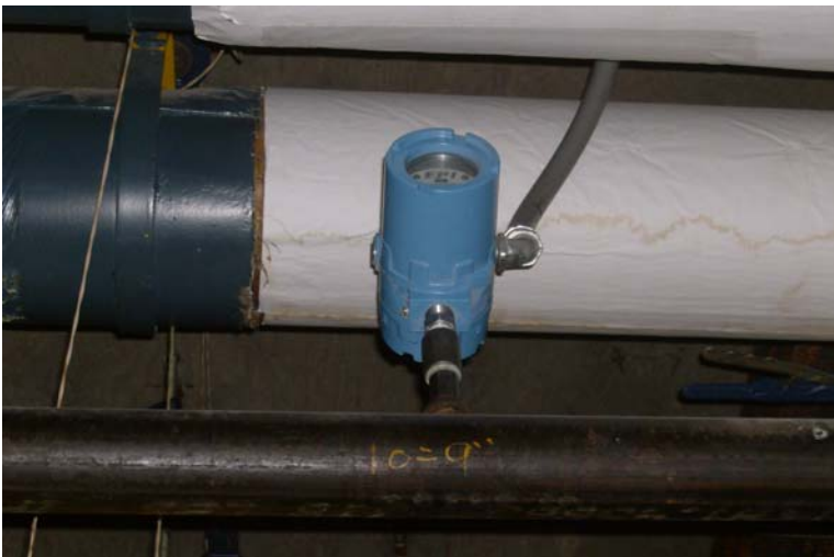
Figure 8. EPI Gas Meter in Mechanical Room
