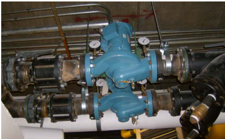
Figure 10. New Hot Water Booster Pumps
