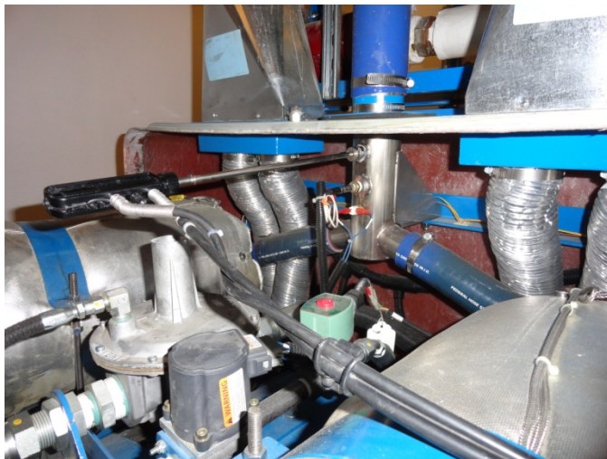
Figure 2. Test Port with Testo 350 XL Probe In Place
