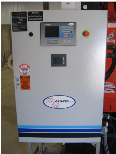
Intelisys Base Box and Digital Power Display
