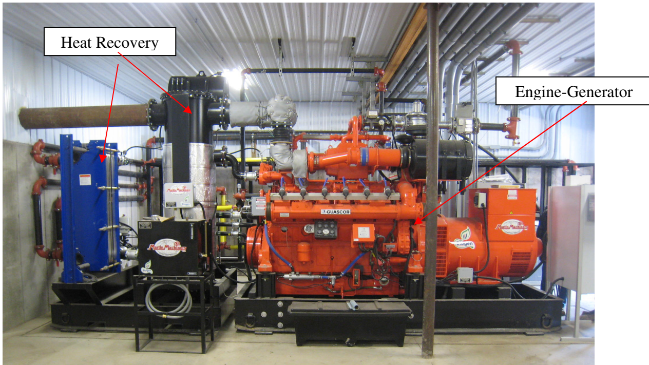
Guascor 5FGLD 360 Engine-Generator and Heat Recovery Equipment
