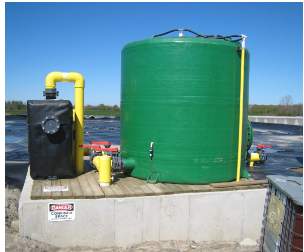
Scrubber and Effluent Tank (H 2 S Removal)
