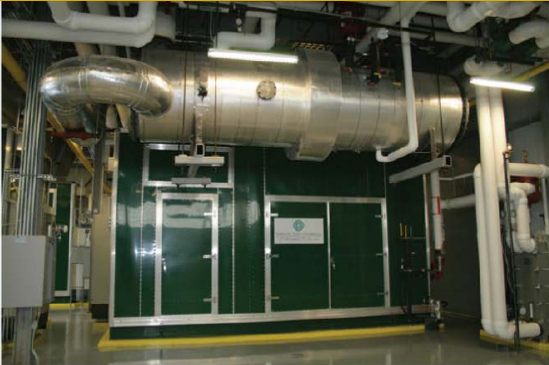
FIGURE 7 ENGINE IN ENCLOSURE WITH HEAT RECOVERY HEAT EXCHANGERS (UPPER FOREGROUND)
