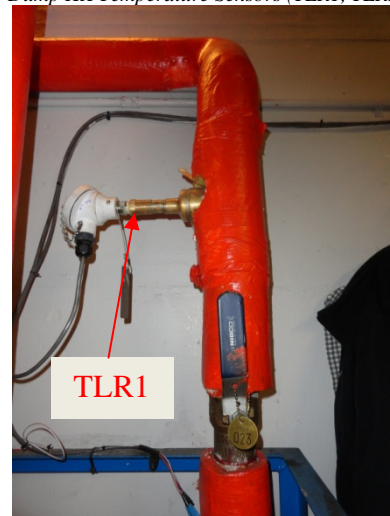
Dump HX Temperature Sensors (TLR1)
