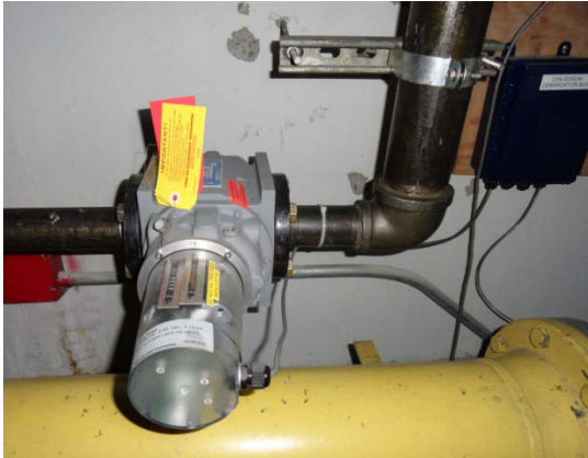
Figure 4. Utility Gas Pulse Output Demarcation
