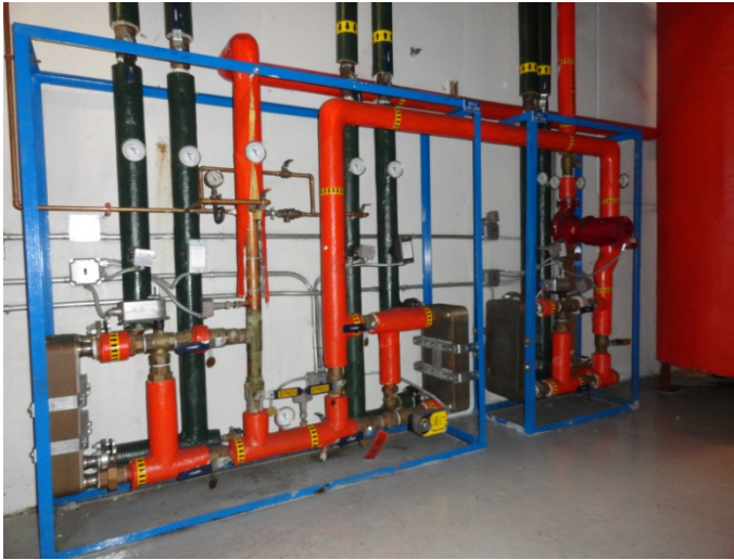
HX-1, HX-2, HX-3 Low, Mid and High-rise DHW HX and Storage Tanks
