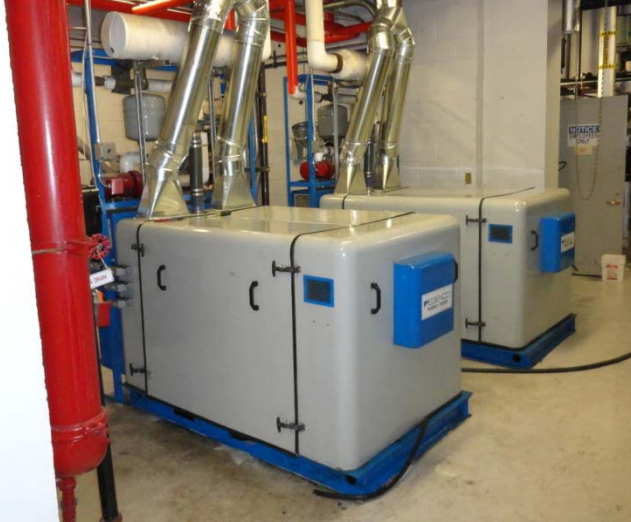
AGEN 75-kW Engine Generators
