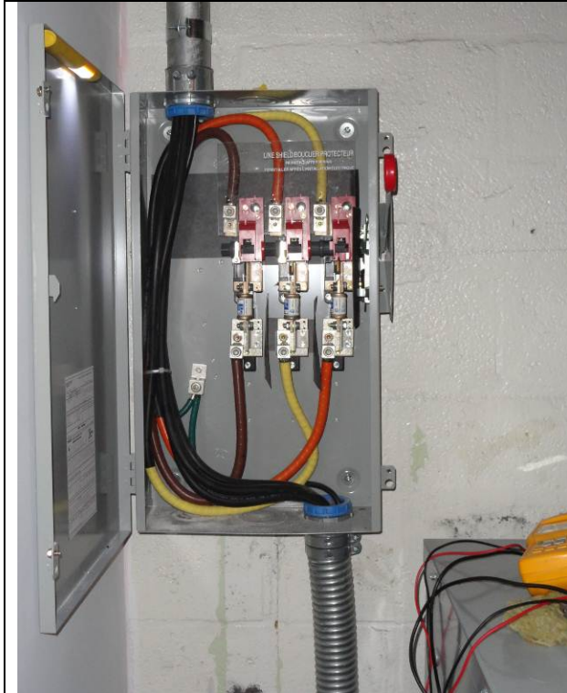
480 V Disconnect – Gross power measurement location
