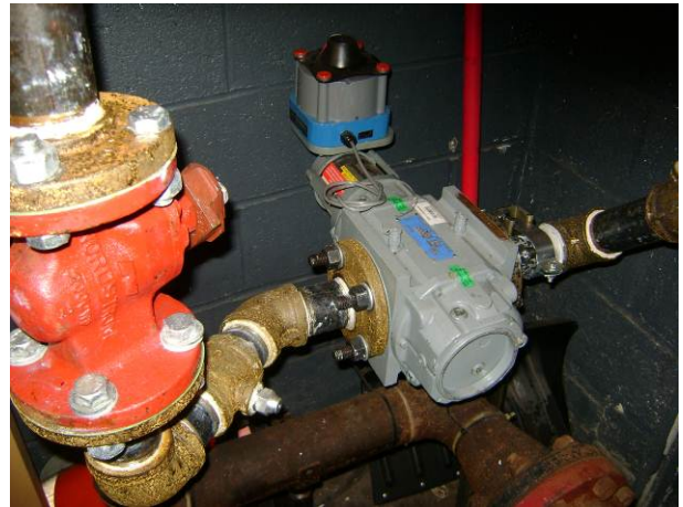
Natural Gas Meter
