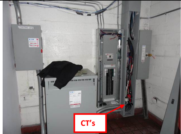
Cogen disconnect (far left) and CT location
