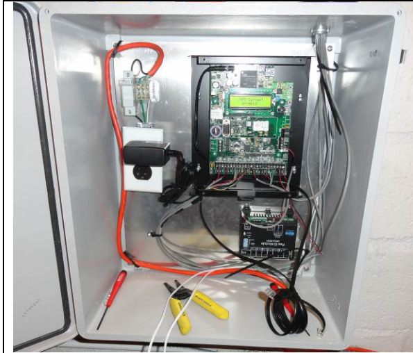
CDH enclosure and datalogger
