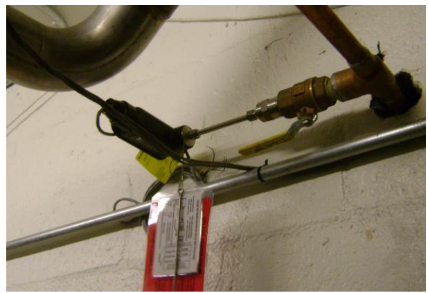
Boiler Loop - flow meter
