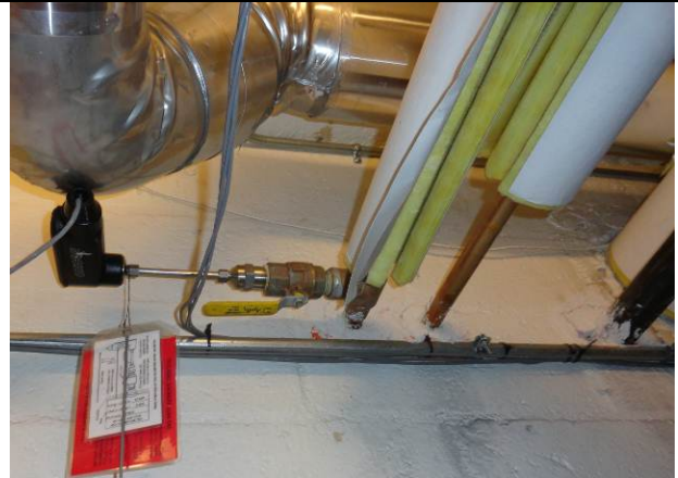
Boiler heating loop flowmeter – FHW2
