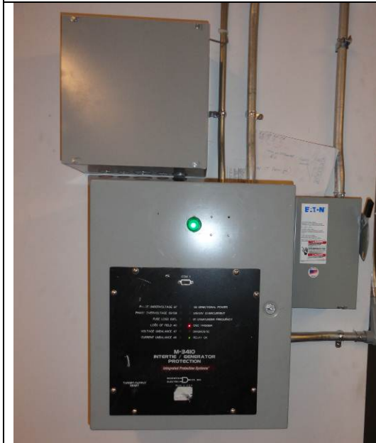
Beckwith panel (bottom) and Wattnode panel (top)
