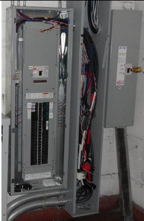
208 V breaker panel (left), 208 V feeder panel (center), and 208 V disconnect (right) – Net power measured in center panel.
