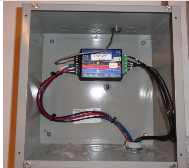
Wattnode inside enclosure
