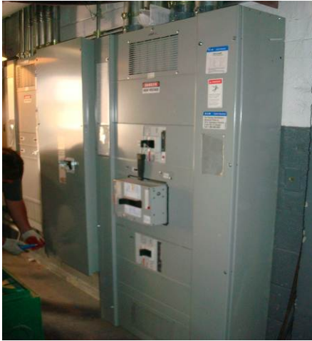
10 th Floor Engine Power Panel
