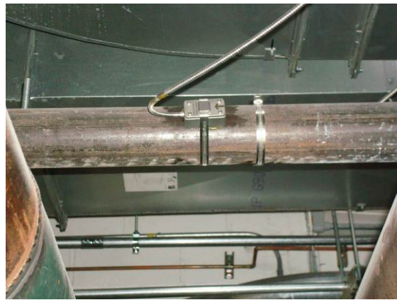
Dumped Heat Flowrate (FM-5)
