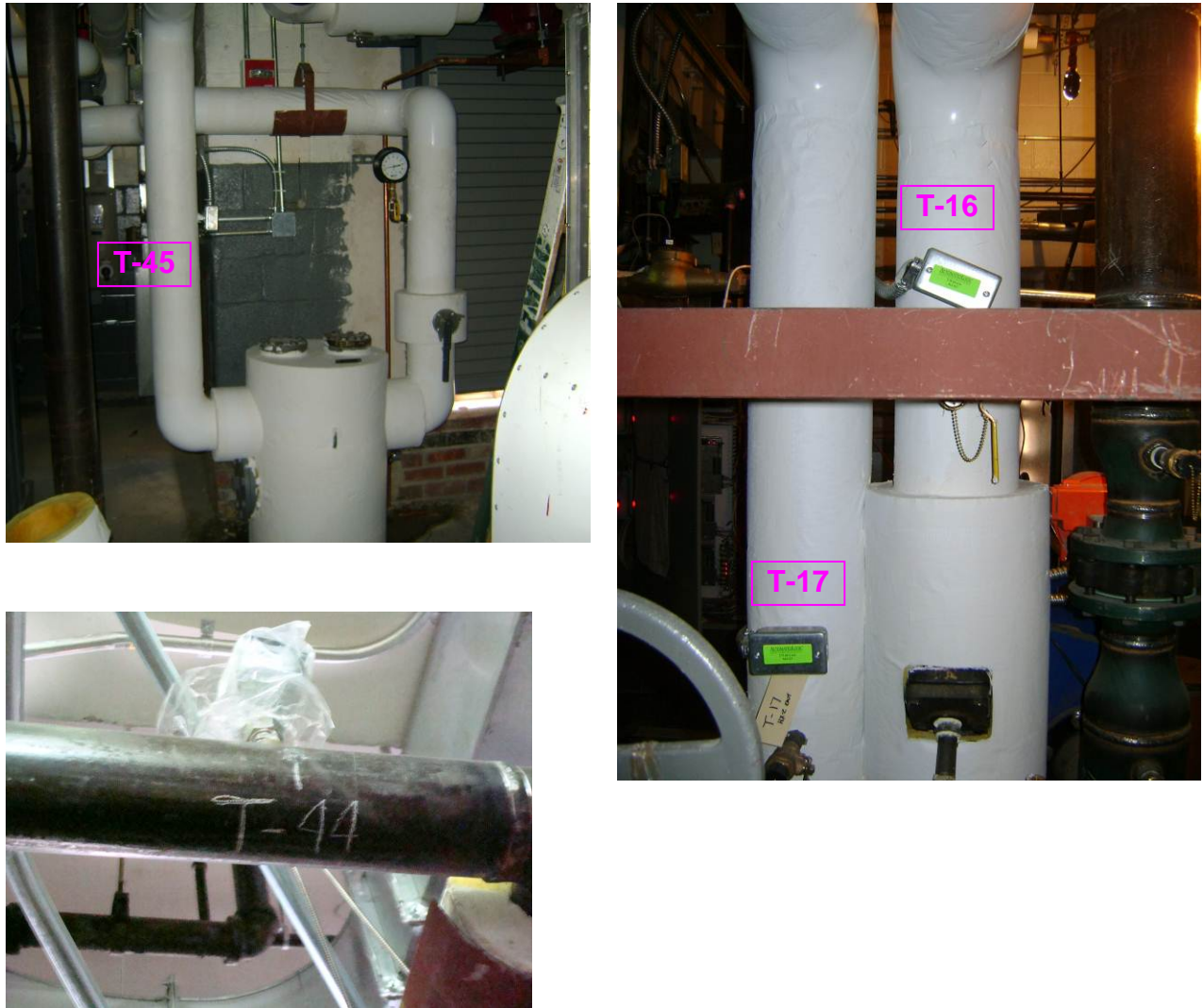
HR Return Temp (T-44) Back to Engines
