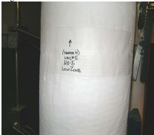
HX#5 - Plumbing Low Zone
