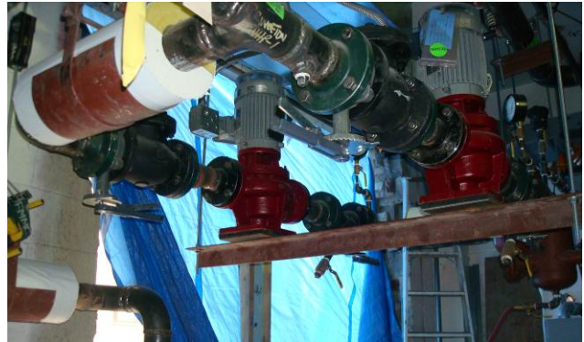
Main Loop Pumps
