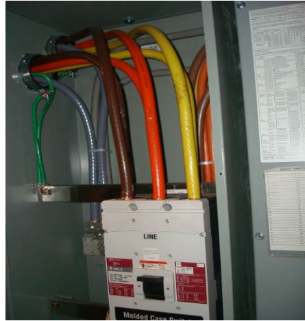
Suggested Location for Power Transducer for Engine Power (WG, 3 engines combined)
