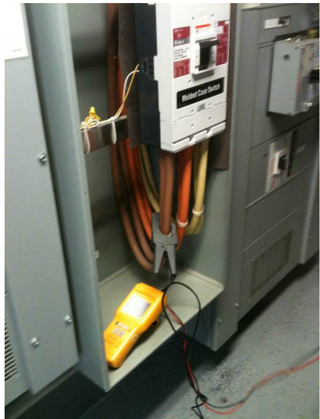
CGDP-2, 800 A cogen disconnect panel. Location of power verification and Veris power meter future location.
