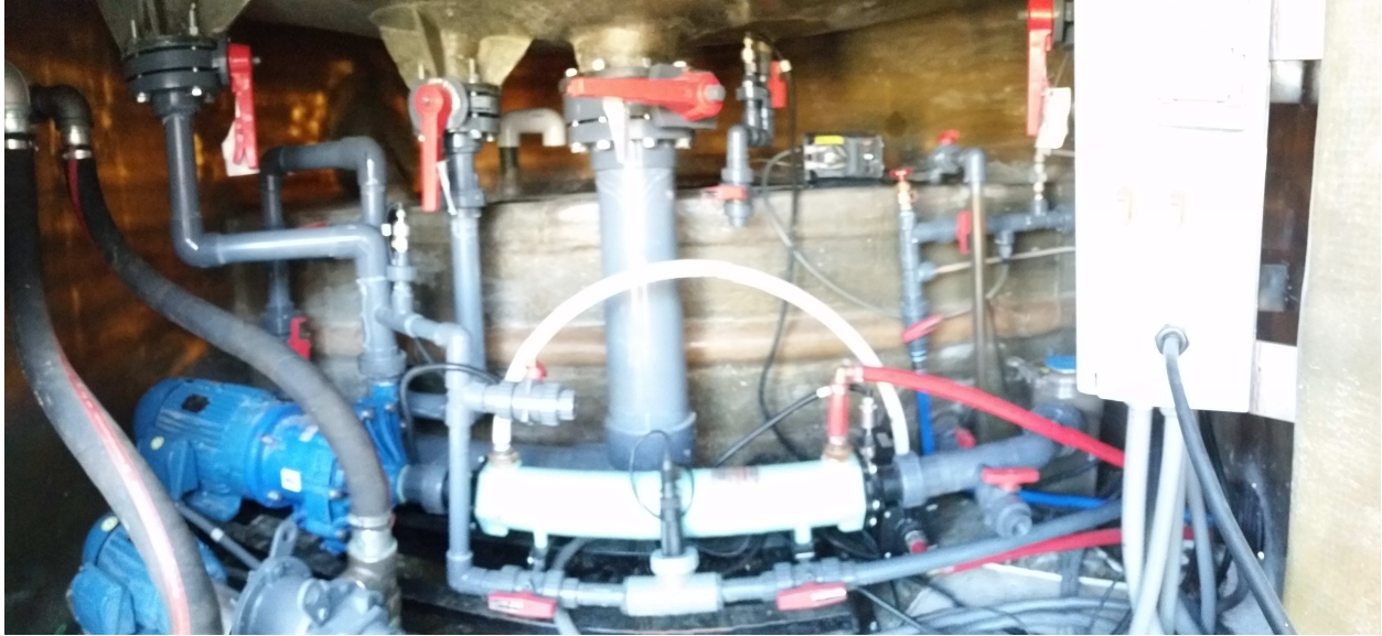
Air Blower & Recirculation Pump
