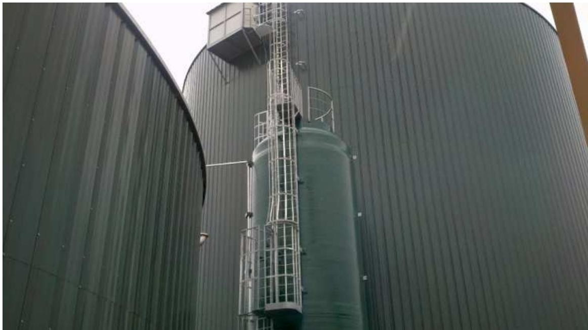
Digester Gas Scrubber and Storage
